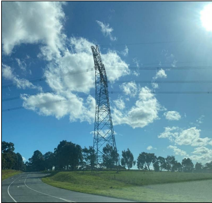
Figure 11 High voltage towers and power lines at the corner of Yarra View Road and Paynes Road
